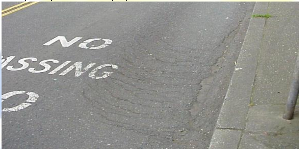
Fig. Slippage Cracks
