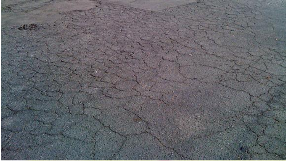
Fig. Alligator Cracking
