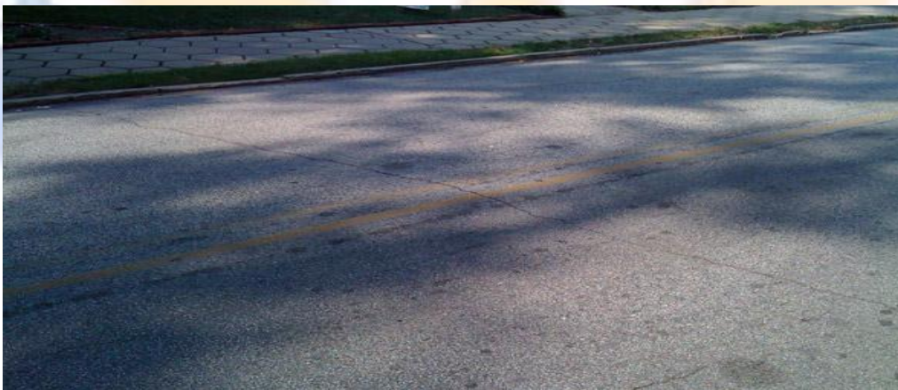
Fig. Transverse Cracking
