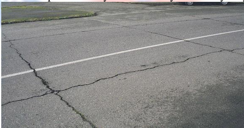
Fig. Joint Reflection Cracks
