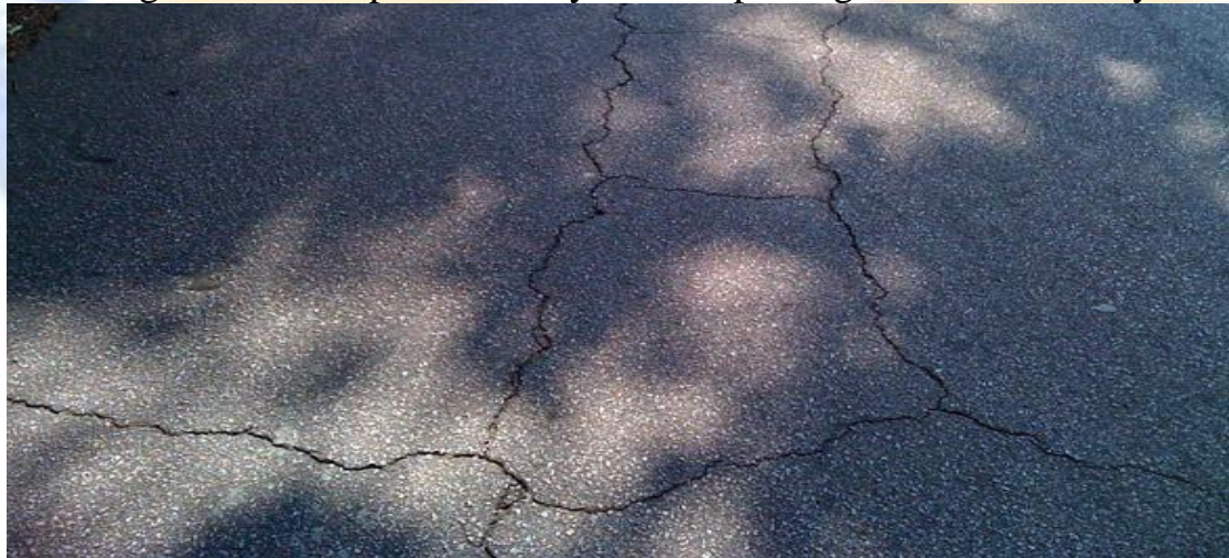
Fig. Block Cracking
