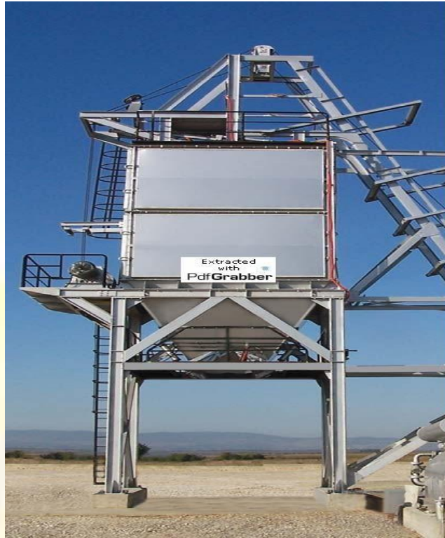
Fig.Hot mix storage silo
