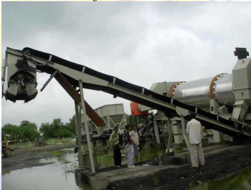
Fig. Load Out Conveyor
